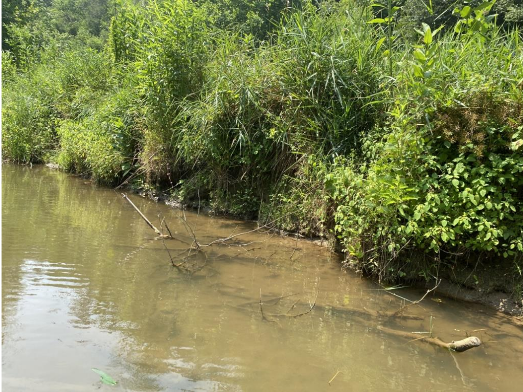
Erosion Area 13; Category “Moderate”
