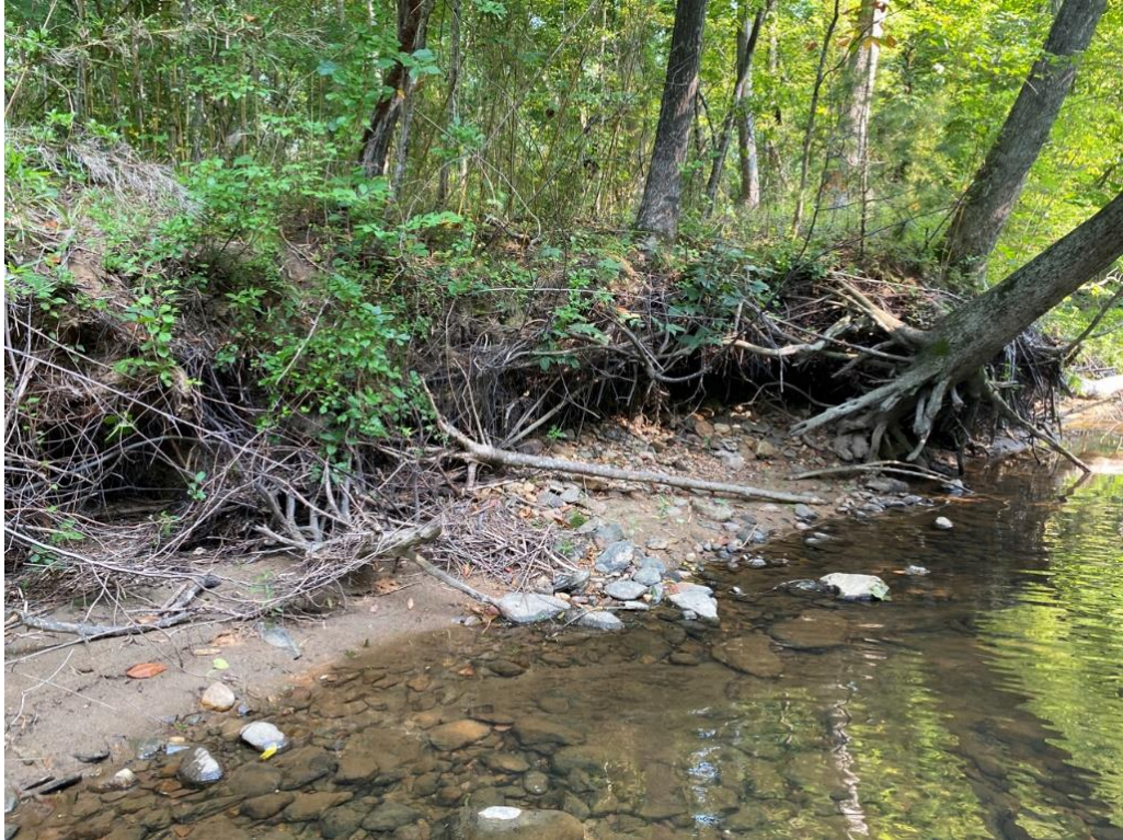
Erosion Area 9; Category “High”
